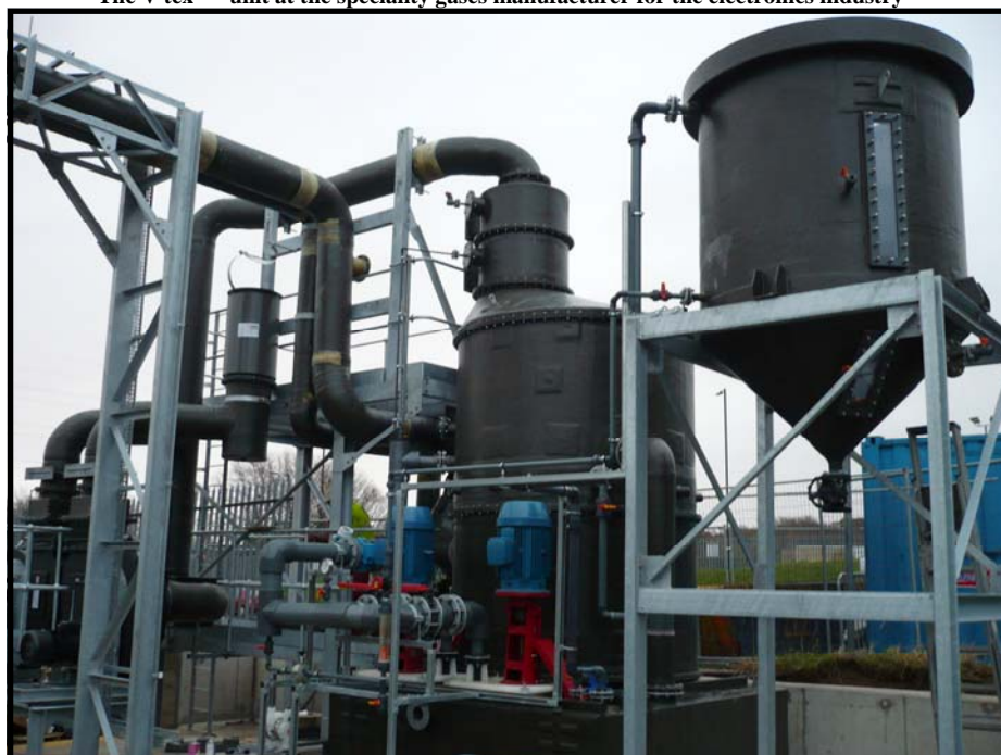
The V-tex™ unit at the speciality gases manufacturer for the electronics industry
