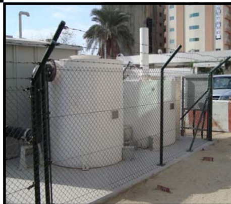
The Ajman water regenerable carbon odour control system
