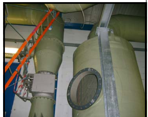
The venturi scrubber and separator at St Leonards-on-Sea
