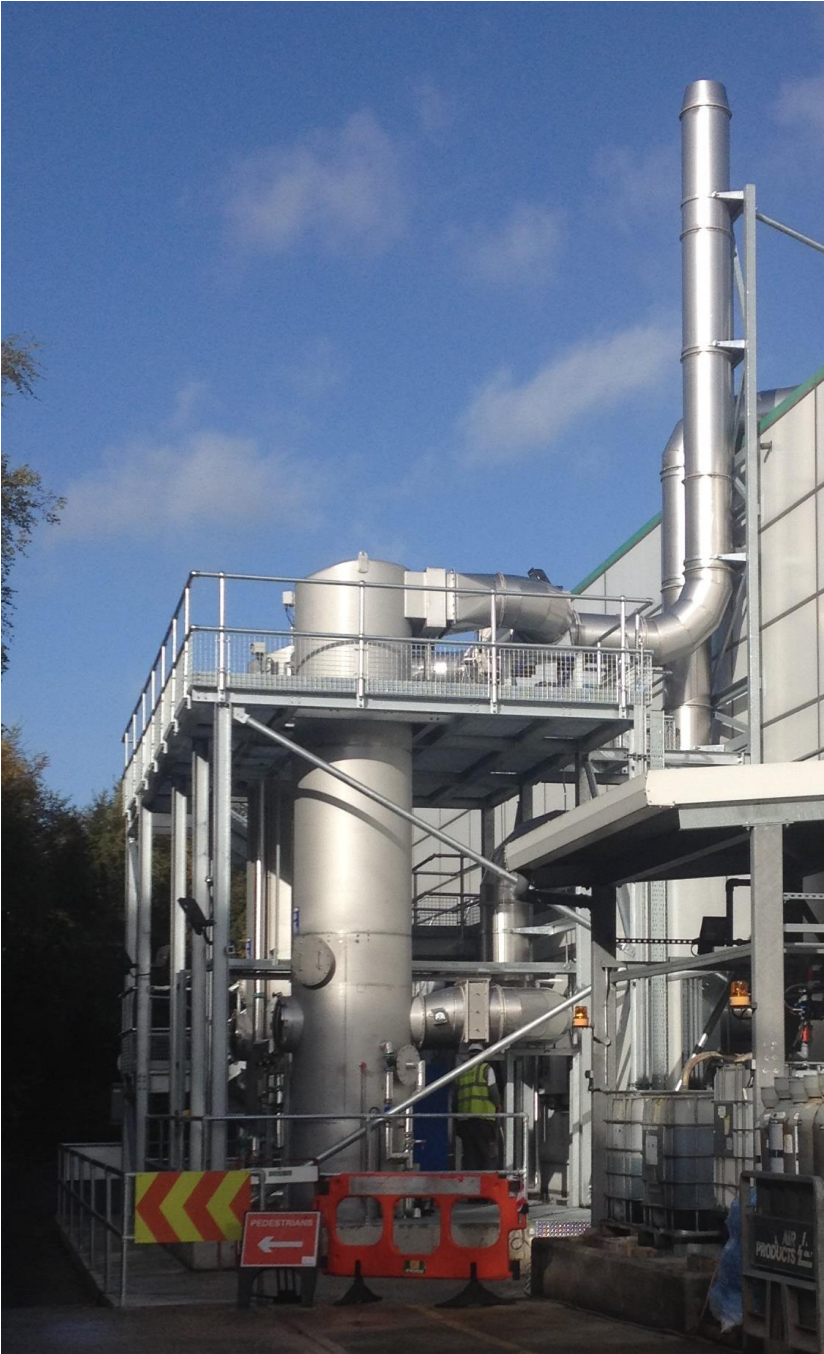
Detail of the completed solvent abatement system in situ
