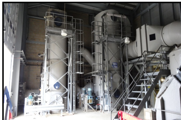
Fig 1 – Scrubbers and demister. Temporary / bypass scrubber on left; new main odour scrubber on right
