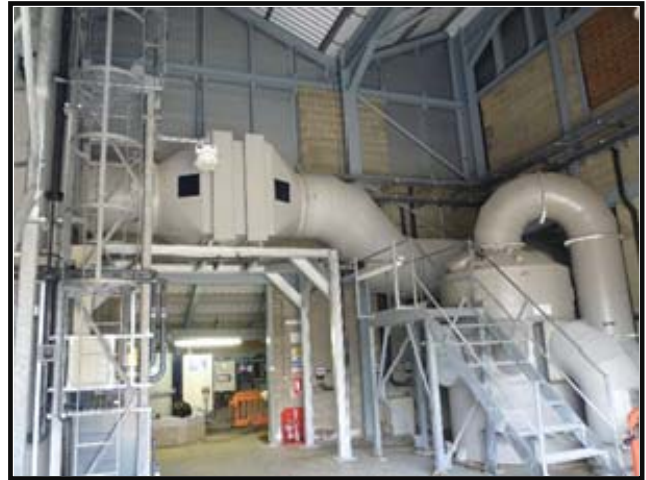
Fig 5 – New demister with support structure and existing carbon filter with access. Chemical storage and dosing room behind
