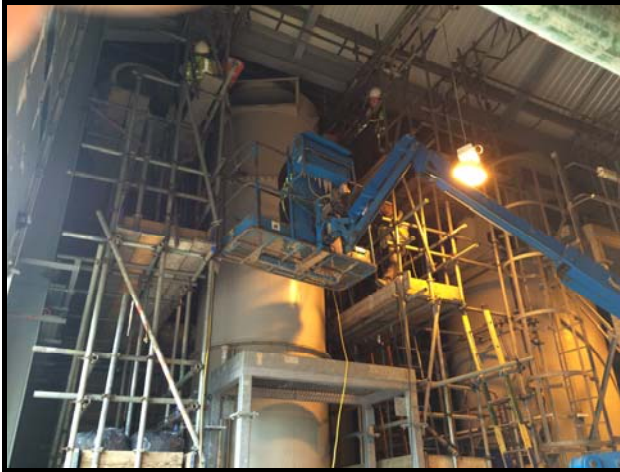
Fig 6 – Modification of original acid scrubber to provide temporary odour control
