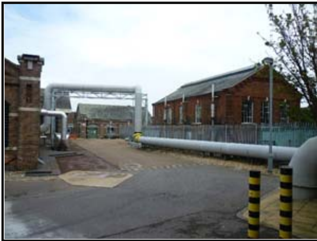
Fig 4 – New pipe bridge and ductwork from detritor and screens area
