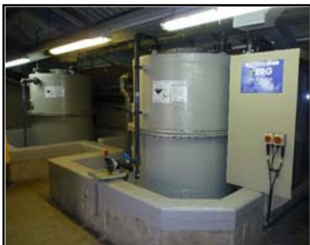
Fig 8 – New bleach tanks in the chemical store
