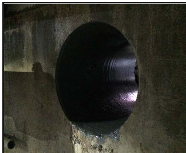
Fig 3 – New penetration through the detritor wall for the new odour control extraction duct
