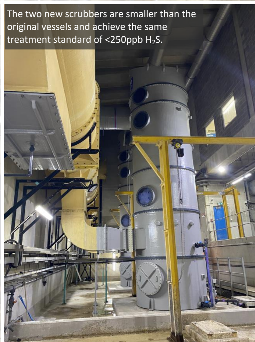
Installing the new ERG OCU involved bypassing the original OCU, cutting up three original scrubber vessels and replacing them with two new, high efficiency scrubbers - extensive scaffolding for safe access.
