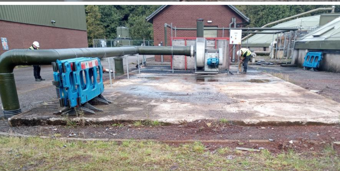
Slab before replacement equipment is installed. Emergency carbon filter supplied by ERG keeps the works functional
